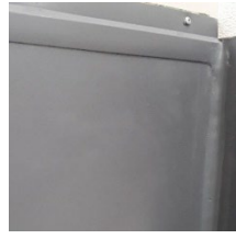
Corner cove on wall
